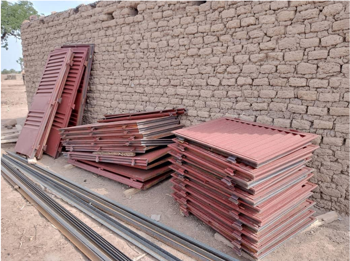
Window and door frames are ready to be mounted. They will be painted on-site.
