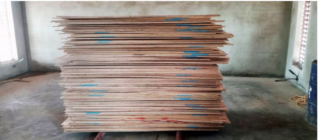
The plaster works inside the classrooms is completed. The wooden panels for the false ceiling are on site, ready to be mounted.
