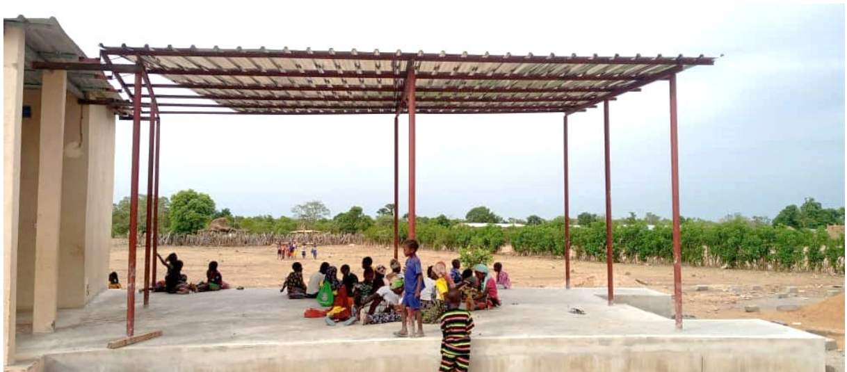
The plastering works of the Façade of the classrooms are completed. The wide roofing also covers the pedestal. The students enjoy already the shadow.
