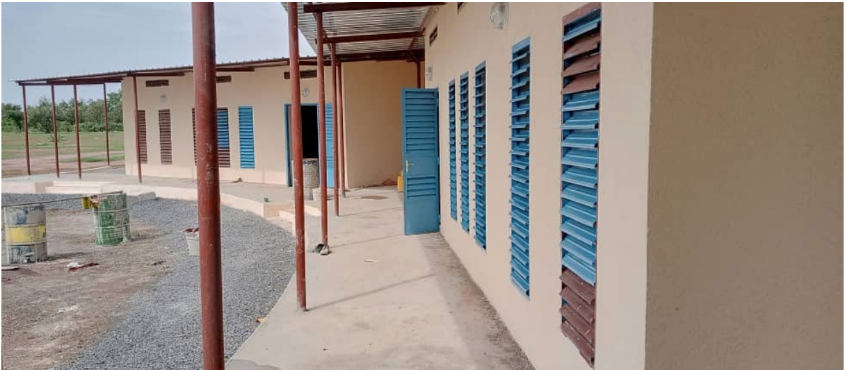
windows, doors, and all the vertical elements that support the roof will be painted blue.
